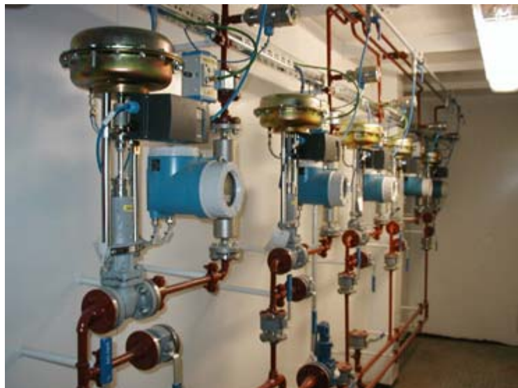
Fig. 8: Measuring and dosing station with pneumatic valves
